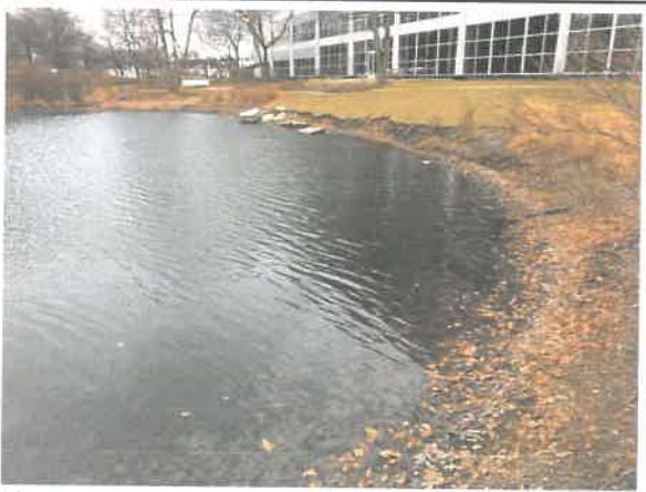
Photo 3: Pond erosion before stone toe stabilization.
