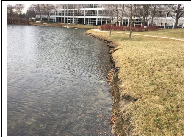
Photo 1: Pond erosion before stone toe stabilization.
