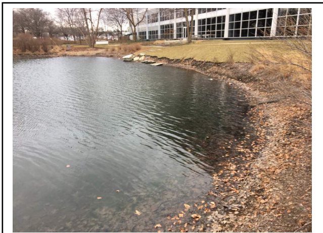
Photo 3: Pond erosion before stone toe stabilization.
