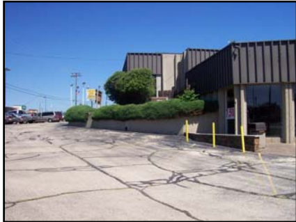
Example of deteriorated improvements (parking lot) located at northeast corner of Route 31 and Sullivan Rd.
