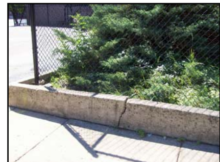
Example of deteriorated improvements (curb) located on John Street
